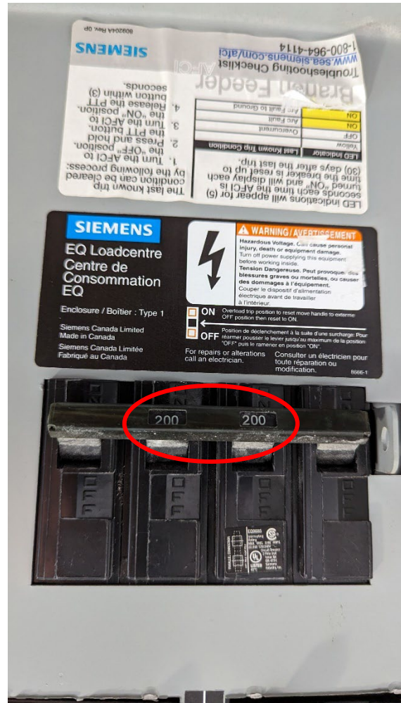
Figure 2 – Panel main switch indicating 200A service
